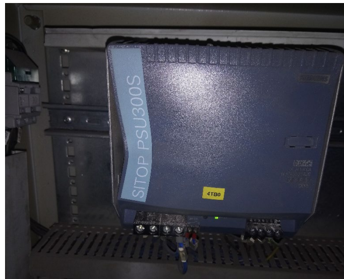
Figure 3 / Heat impact on an I/O box which remained open during scrap charging
